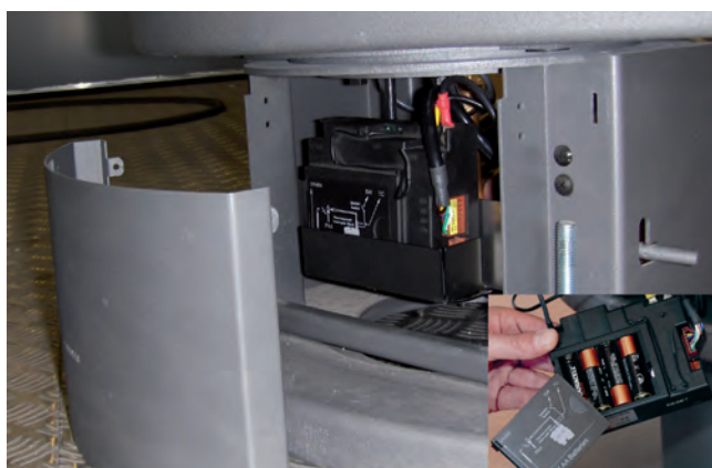
Replacing the batteries of the receiver.
