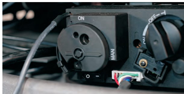
The gas control switch
