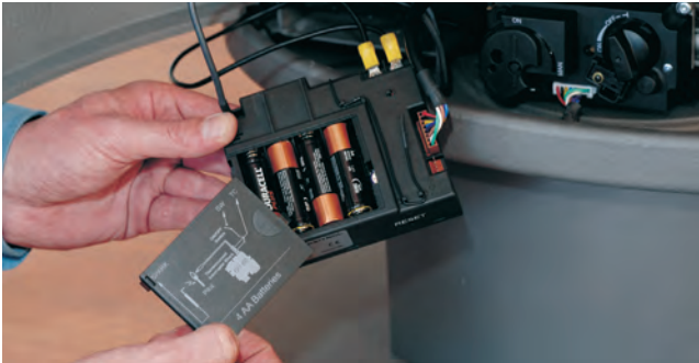
Replacing the batteries of the receiver.
